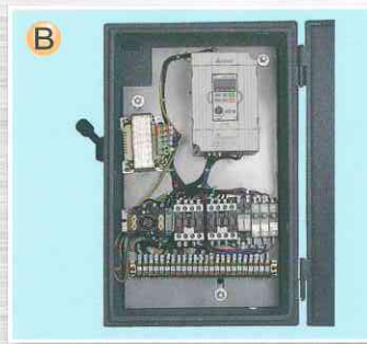
■ Safety Electric Box with Inverter
